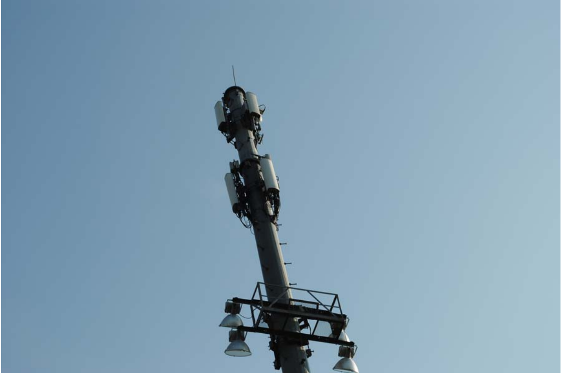
Figure 3: T-Mobile Beta Sector Antennas #5 through #7 - Below
