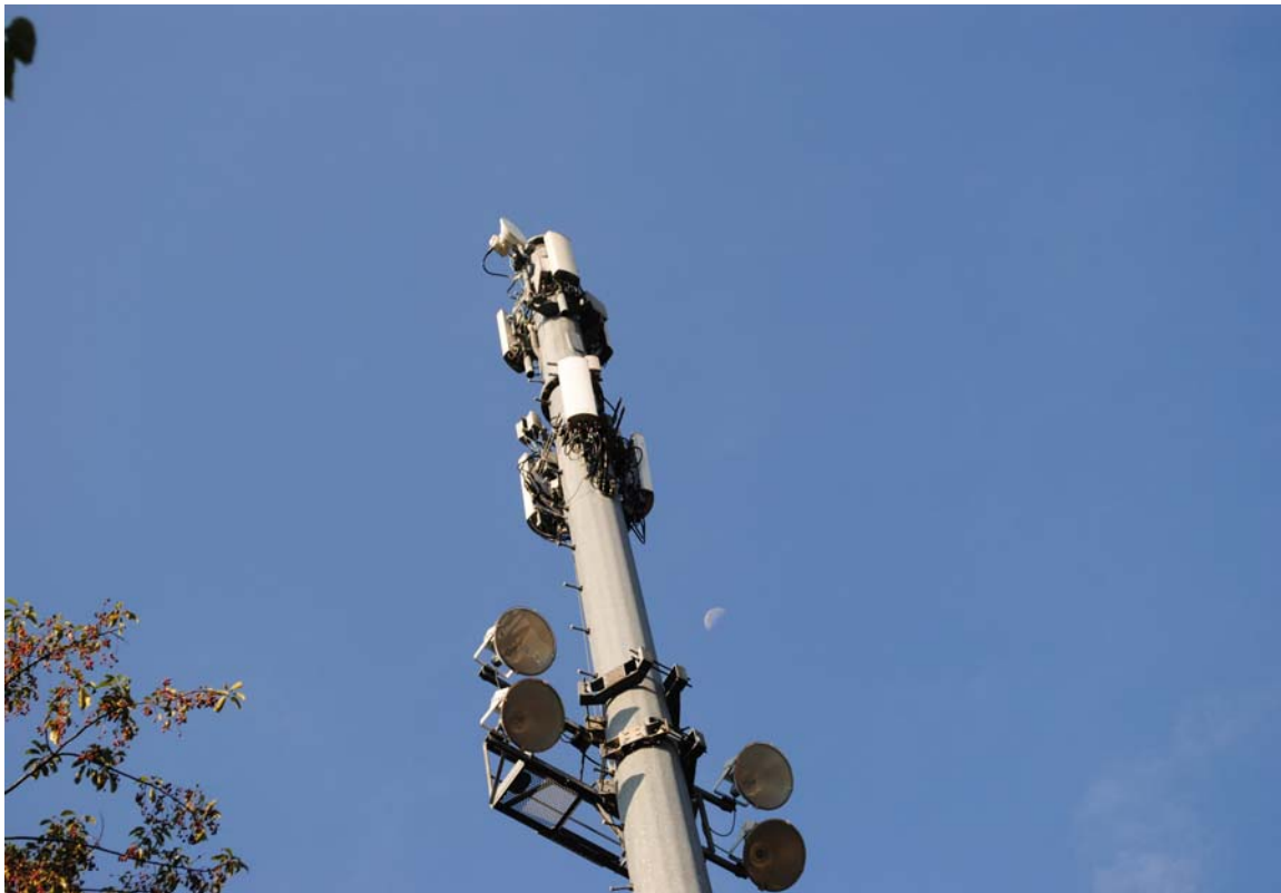
Figure 2: Clearwire Sector Antennas #1 through #4 - Top
