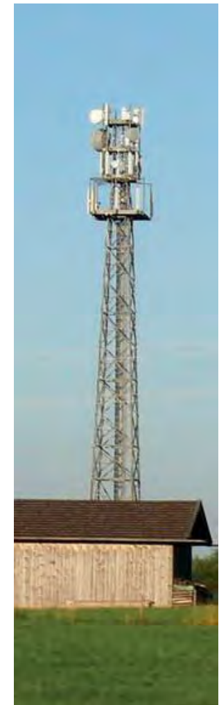
Mobile phone mast Seehausen (686 m / 2250 ft above sea level) Height: 36.1–43.8 m, 36 antennas (2020)
