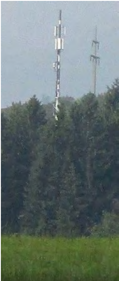
Mobile phone base station of Rickenbach, view from south, from forest edge
